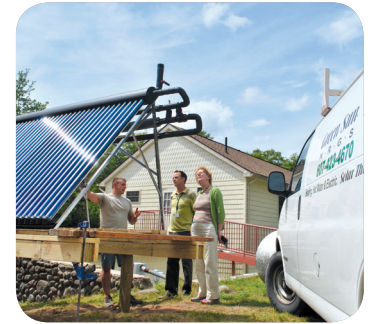
Solar Thermal System
